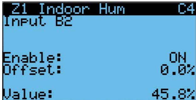
FIGURE 42 Enable/Disable Zone 1 Indoor Humidity Sensor
