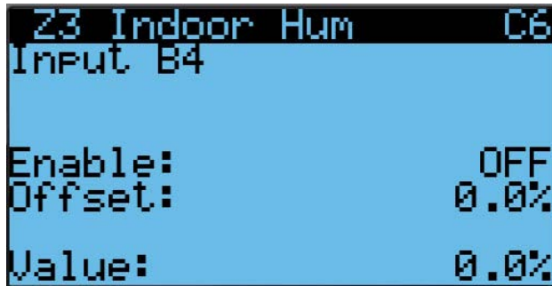
FIGURE 44 Enable/Disable Zone 3 Indoor Humidity Sensor
