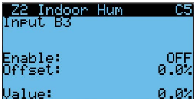
FIGURE 43 Enable/Disable Zone 2 Indoor Humidity Sensor
