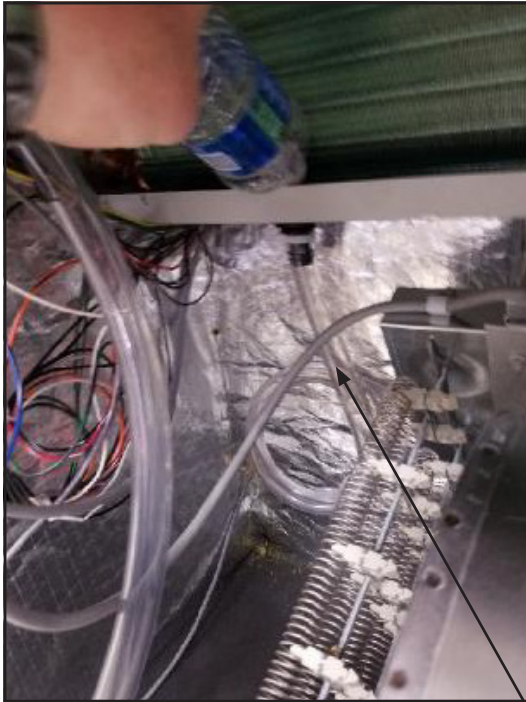
Evaporator Drain Pan Left Side Drain Hose
